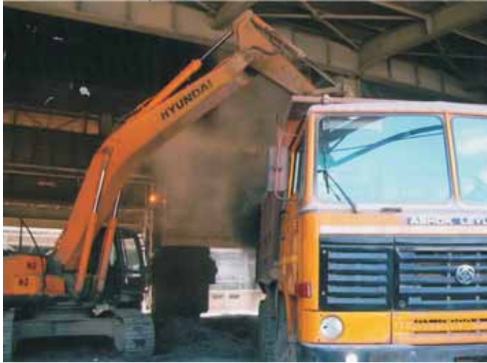
BIGGER SIZE EXCAVATORS IN OPERATION FOR EXCAVATING OF HOT SLAG & TRANSPORTATION OF HOT SLAG AT JINDAL STEEL WORKS LTD. (JSW)
