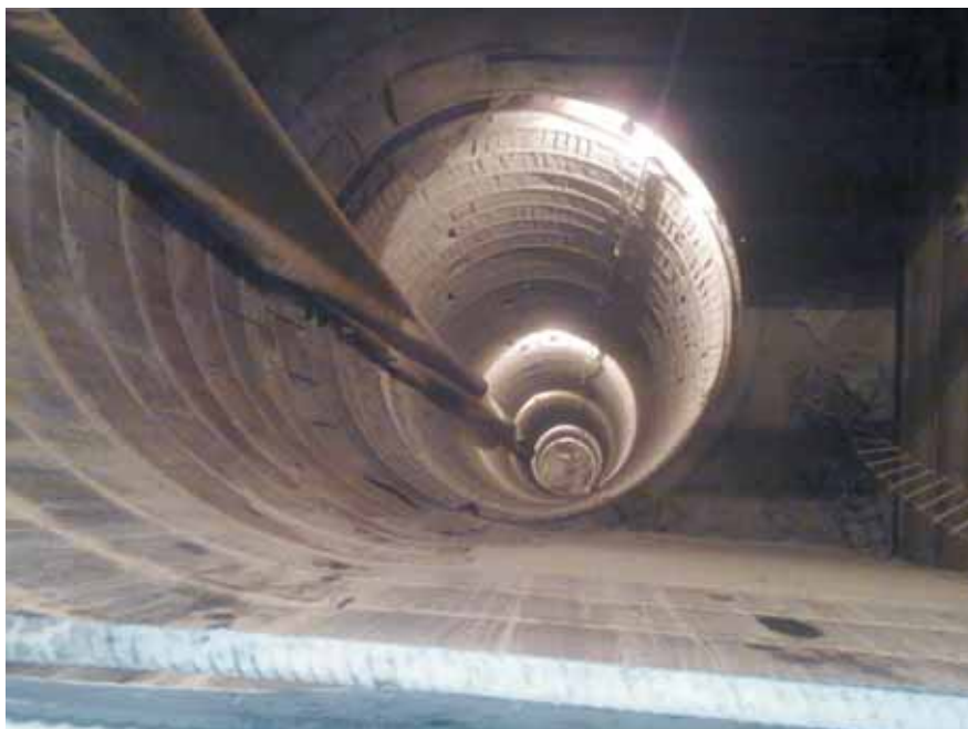
Vertical Pressure Shaft of 5.2 Mtr Dia and Height of 165 Mtrs. With complete RIB Support.
