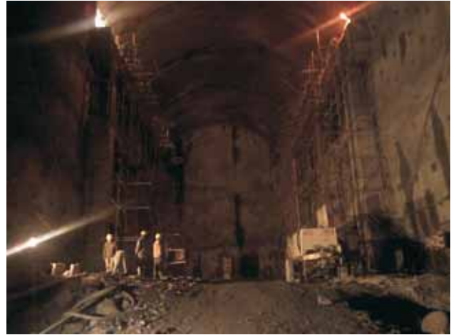
Power House Cavern Service Bay Gantry Crane structures.
